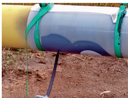
Fig. 5: Discharging ahead of the flow front
